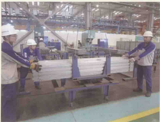
● 吊车未给信号起吊
