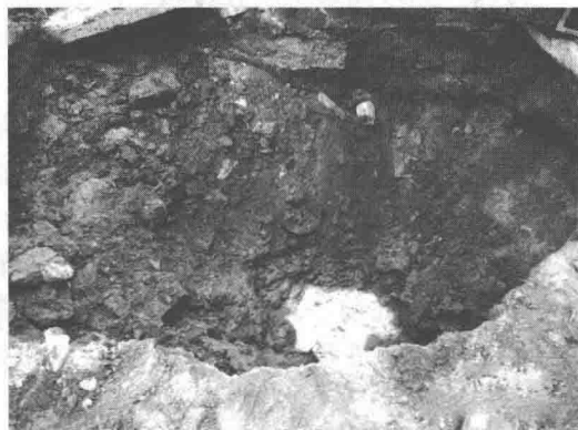
(b) 护壁坍塌
