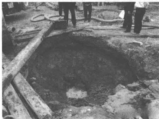
(a) 成孔时坍塌
